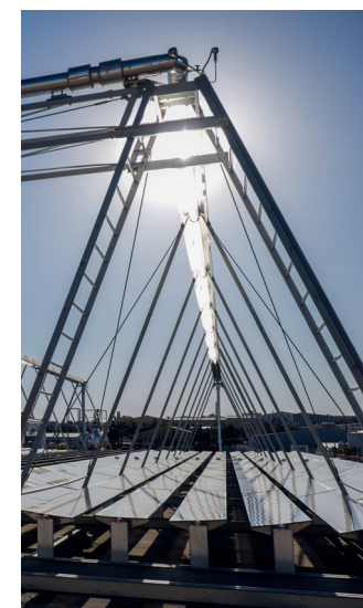
2. Linear Fresnel Reflectors at RAM plant in Jordan (source: Industrial Solar)
