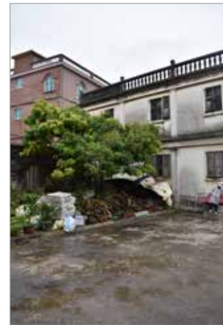
Fig. 2 - One of the abandoned buildings in Dongda village: the space of the patio damaged by incongruous elements (sink and pipes informally added)
