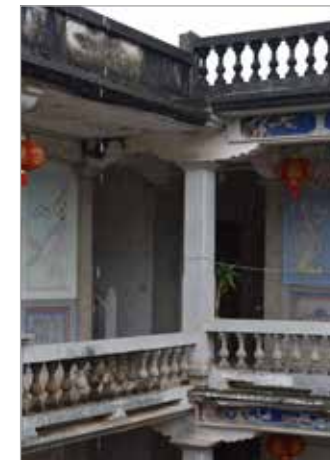
Fig. 3 - One of the abandoned buildings in Dongda village: corner solution of the internal patio, with the detail of the canal-cornice on the top that flows the water from the roof to the patio circulation system passing through the hollow reinforced concrete pillar
