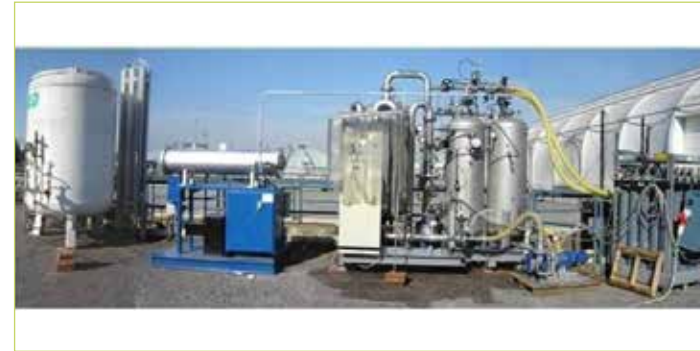
1. View of the ozonation pilot plant: generator (left) and reactor (right).
