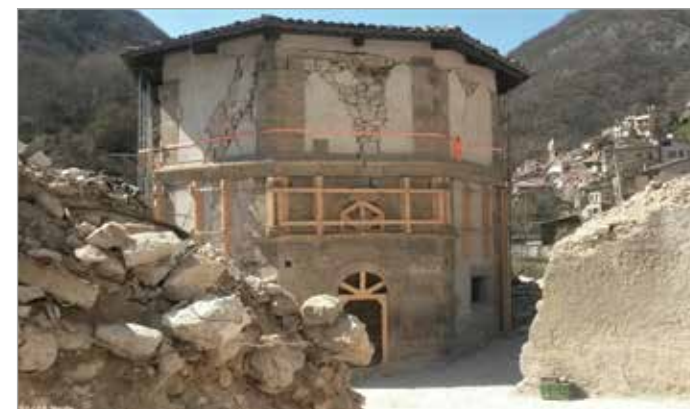
Fig. 1 - The church of 'Madonna del Sole' in Capodacqua, Arquata del Tronto (AP). The technical countermeasures executed in October 2016 increased the residual capacity of the building, reducing the progress of damage due to the aftershocks
