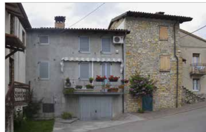
Fig. 2 - State of conservation of widespread heritage in Menconico (PV). On the right, the building has undergone a total scrape of the plaster; on the left, a large opening has been opened to create a garage on the ground floor and the plaster has been replaced with a plastic material. Both buildings have been replaced the roofs and the shutters (photo taken in 2019)
