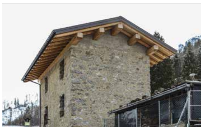
Fig. 1 - The replacement of a roof of a rural building in Valtorta (BG). The roof, although the wooden material, appears out of portion compared to the structure below (photo taken in 2018)
