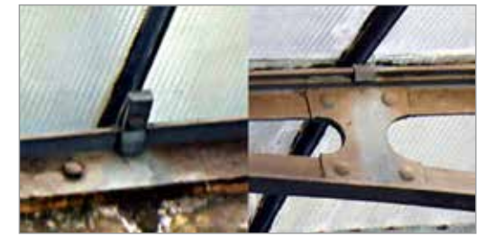
3. Expansion joints that were introduced in the post-war reconstruction of the roof.
