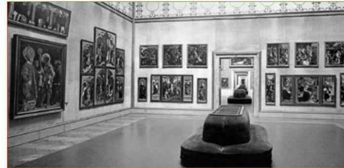
1. An ‘enfilade’ of radiators hidden by seats at the Alte Pinakothek, Munich, in a 1926 picture
