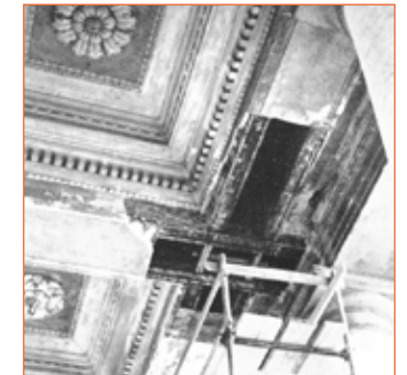
3. Overview of the coffering of Palazzo Chiericati's Doric loggia during the restoration in 1964 (© CISA "Andrea Palladio")
