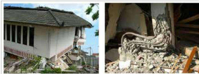
Fig. 1 - Collapse of a residential building in Yogyakarta, Indonesia, after an earthquake in May 2006.
