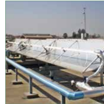
2. The second experimental setup installed on the roof of the Moroccan dairy factory.
