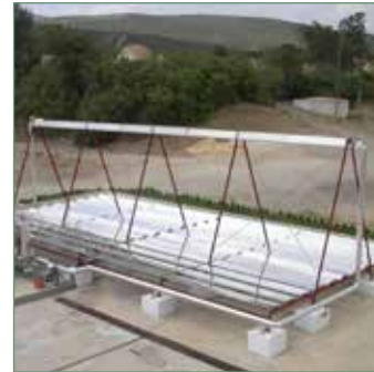
1. The first experimental setup in Tunisia: the solar collector, the absorption chiller and the cold storage.
